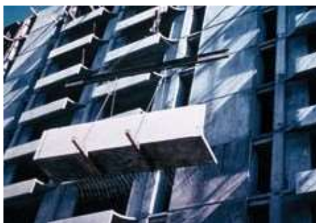
Fig. 2(a). Lifting roof parapets into place on the Queen Emma Gardens building in Honolulu.
